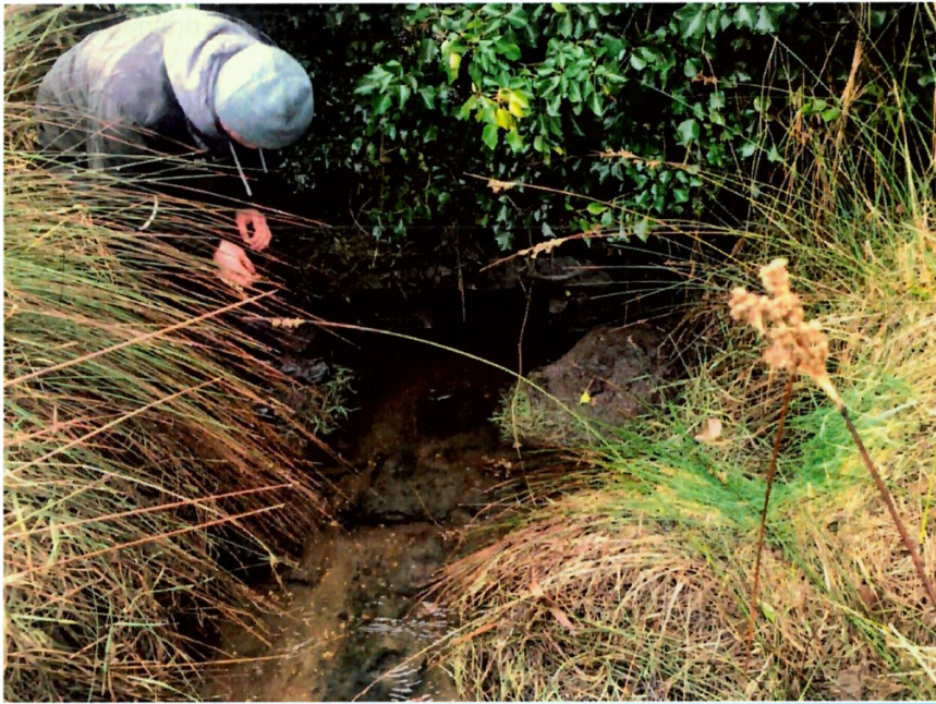
Figure 3 Image of surface water flowing into the existing culvert which crosses the existing R172 Regional Road
