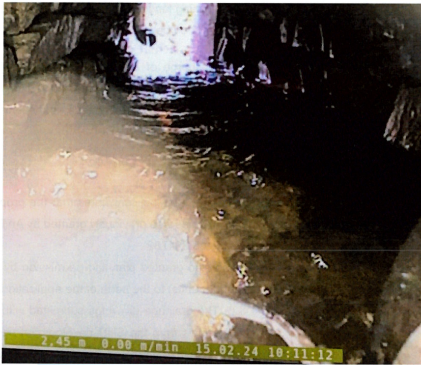
Figure 5 Image from within the existing culvert which crosses the existing R172 Regional Road
